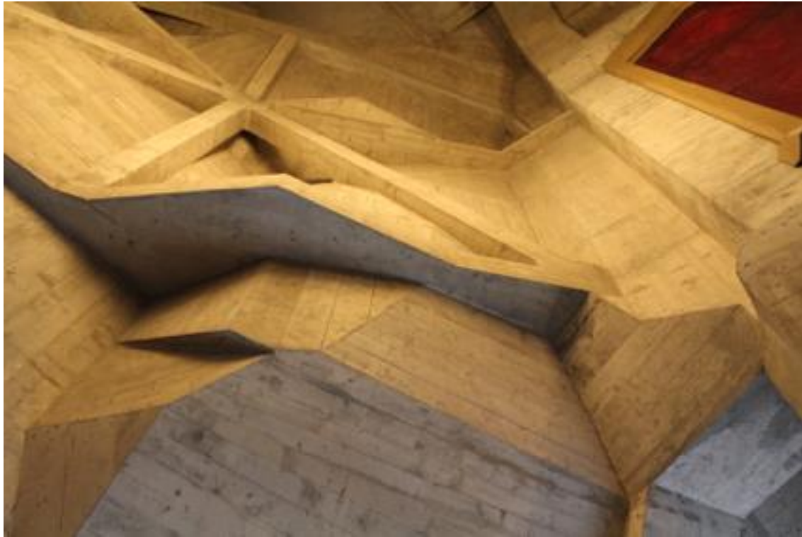
Fig. 7. Goetheanum interior, showing impressions on the concrete of the timber shuttering (formwork) (image: J.Paull).
